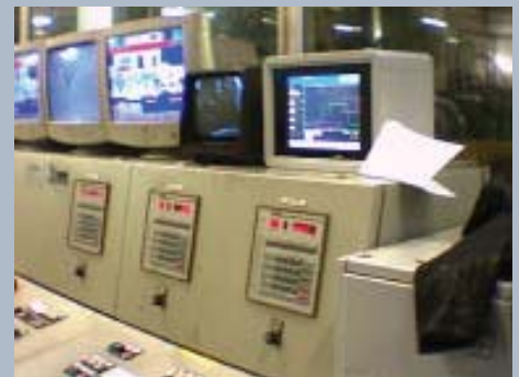
260 Unit mounted on the main control panel.
